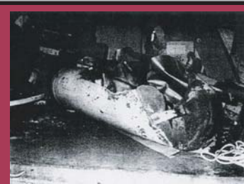
Hot water tank after explosion
