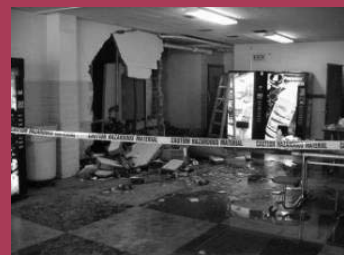
Collapsed wall after the explosion
