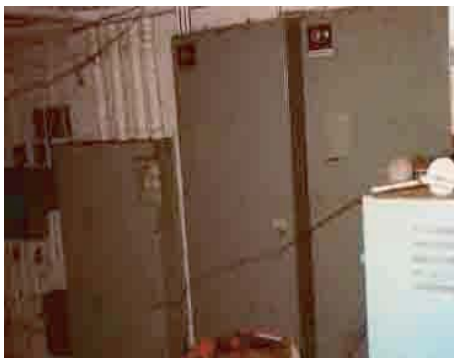
Motor starters submersed in salt water
