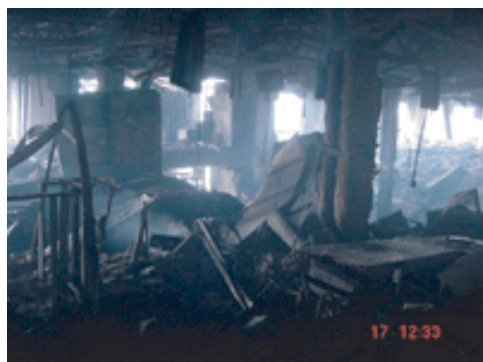
This image was taken by retreating fire personnel as they left the partially collapsed 35th floor
